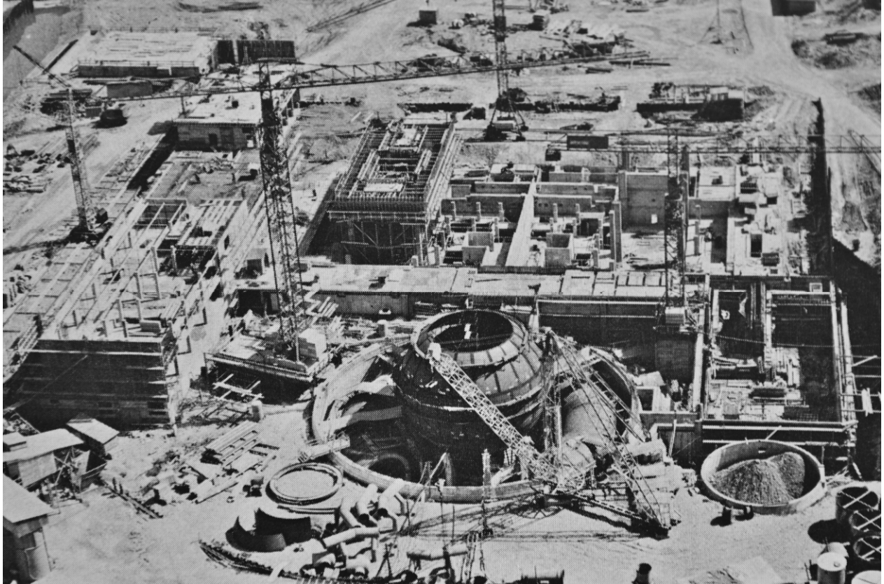
Fig. 1 Construction site from south-west, August 1968. Source: Staatsarchiv Bern, N. P. Böhm 14. Photo: BKW
